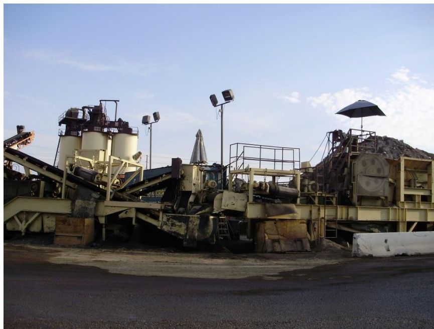
Figure 2-19 Escondido Asphalt Manufacturing Plant
