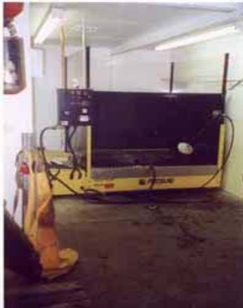
Figure 2-1. Pressure Island Cleaning System at AH Plating.
