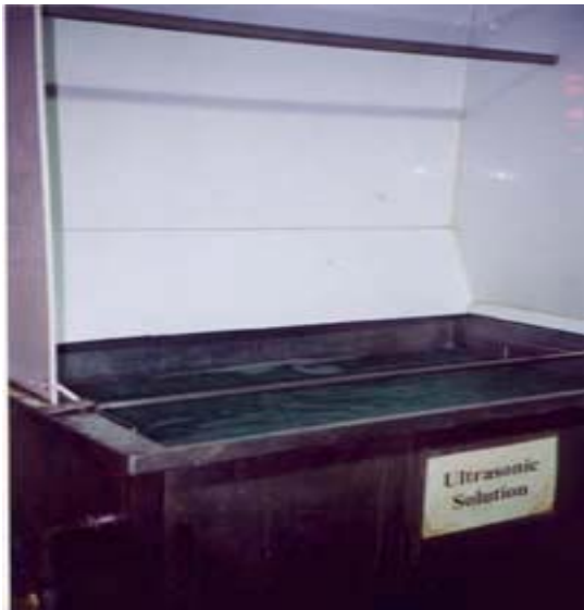
Figure 2-6. Top view of Ultrasonic Unit at Anodyne.
