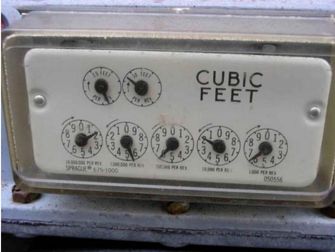
Figure 3-12. Gas Meter Used for the Gas Measurements
