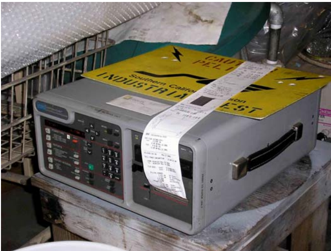
Figure 3-13. Monitor Used for the Electricity Measurements
